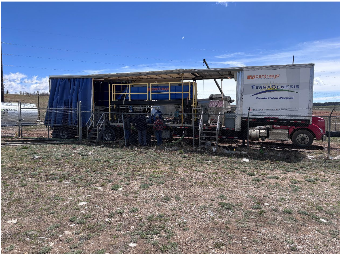
Photo 2: TerraGenesis sludge processing unit
