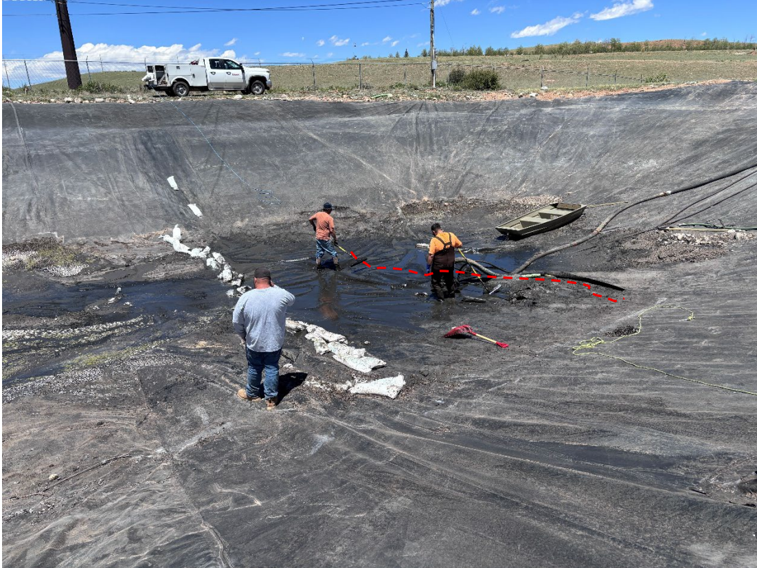
Photo 4: Bottom of the lagoon showing the location of the tear. The dashed line is the approx. extent of the tear.
