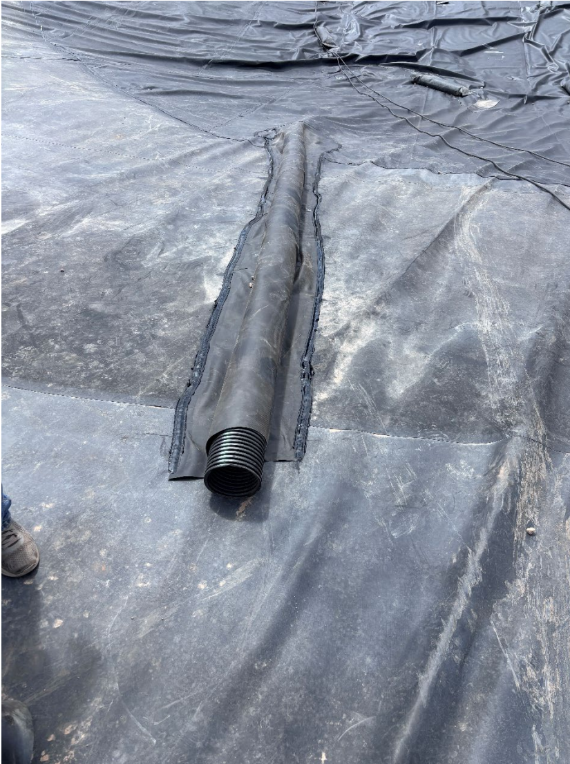
Photo 11: Access point for pumping groundwater from under the new liner
